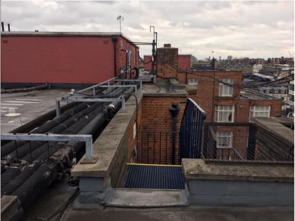
One of the two external Access stairs which lead to roof level
